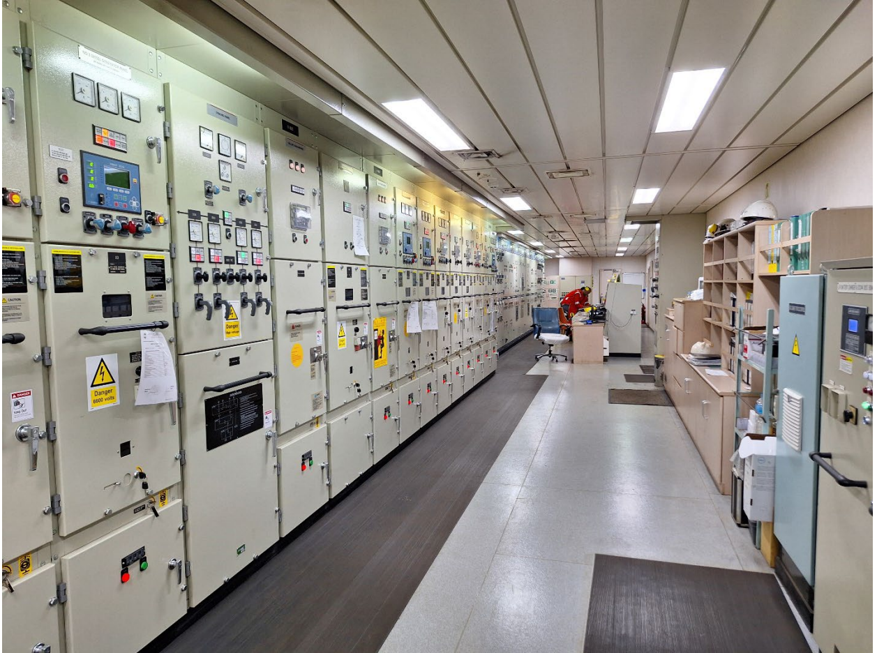
Fig. 2. The Vessel's HV switchboard (located in the Engine Control Room).
