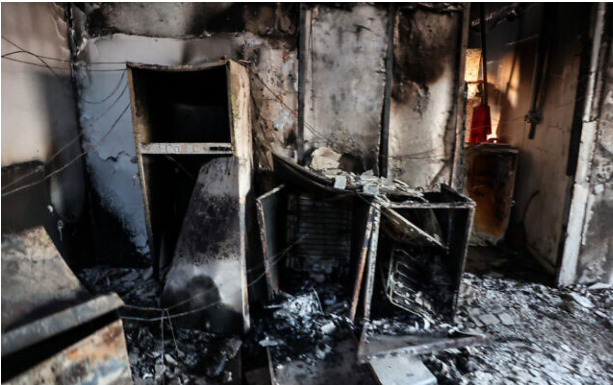
Charred debris and objects are scattered inside a building in Kibbutz Alumim, following the October 7 attack by Hamas terrorists, in southern Israel near the Gaza Strip on October 18, 2023. (Gil Cohen-Magen/AFP)
