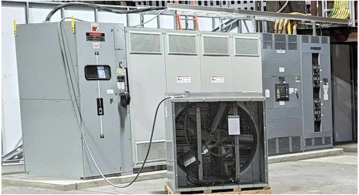
T3 Gear - Minus Transformer
