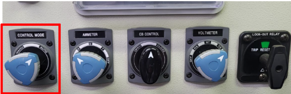
Step-down transformer controls, with the Auto/Manual Control Mode selector at far left. This photograph was taken post-accident.
