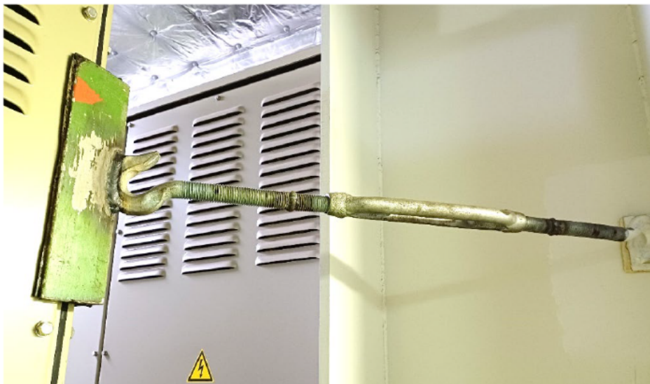
Cargo chain turnbuckle, welded to angle iron, and wedged between the number 1 step-down transformer (left) and a steel beam (right).
