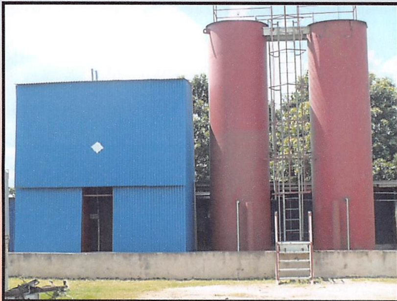
SOLVENT BLENDING FACILITY
