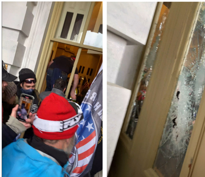
Images 2 and 3: Screenshots from Exhibit 300 showing people climbing through a broken window (Image 2, at 6:38) and the broken Senate Wing Door (Image 3, at 6:48)
