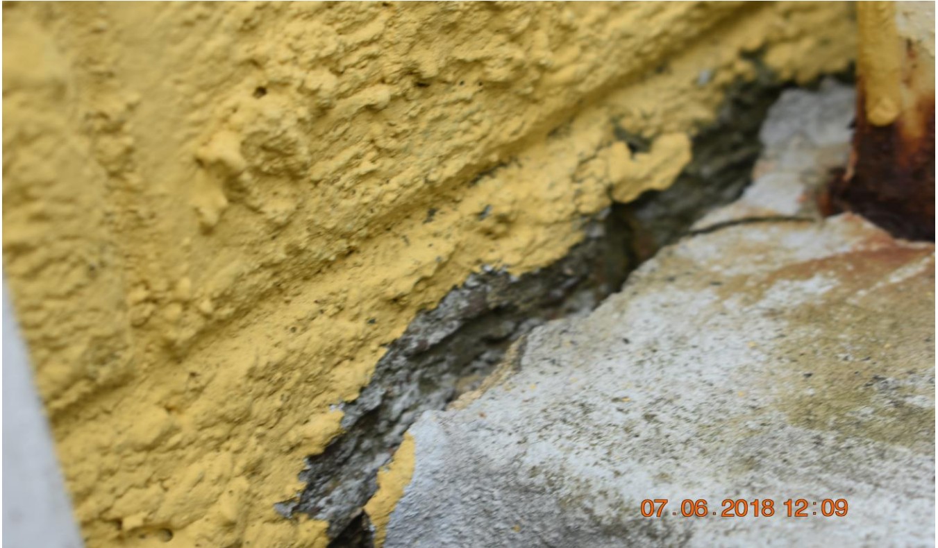
Areaway retaining wall separation
