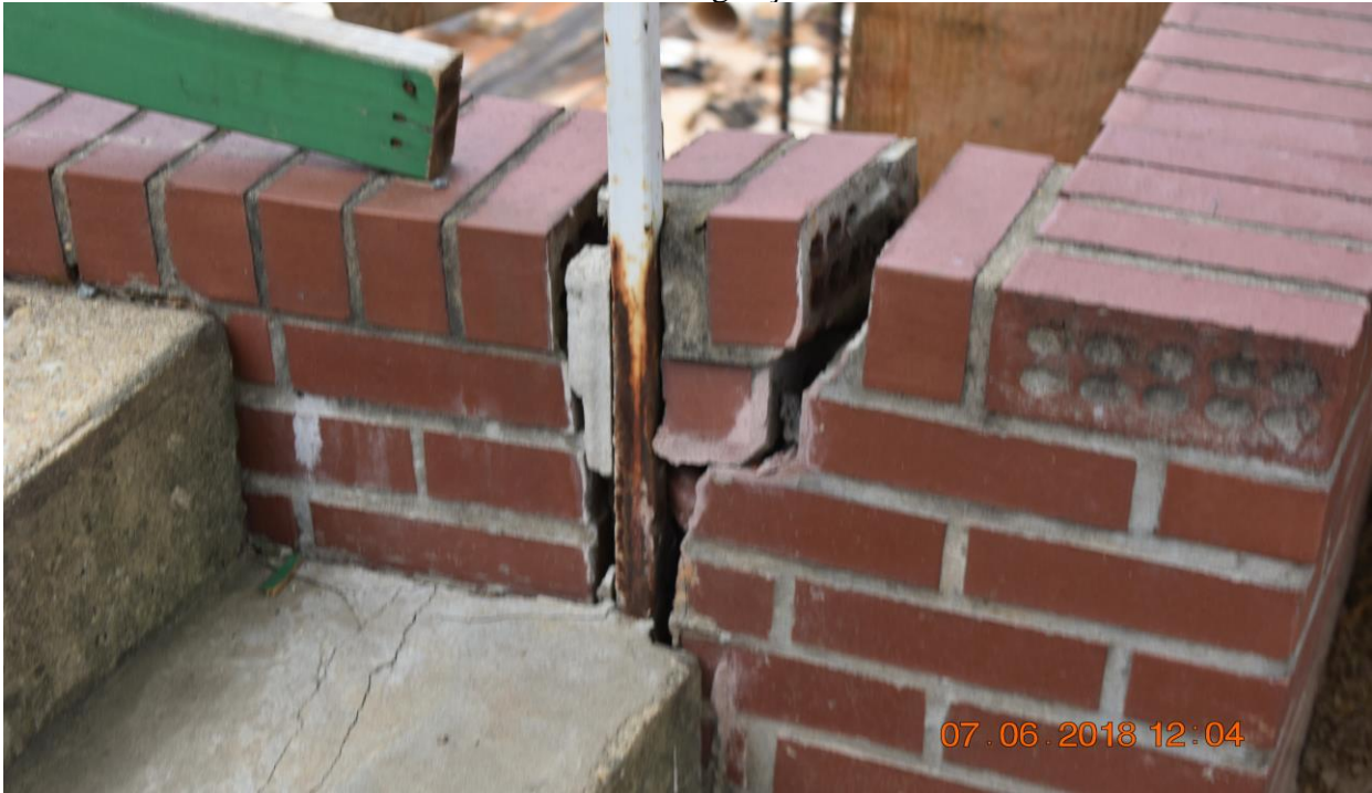
Crack landscape wall at sidewalk
