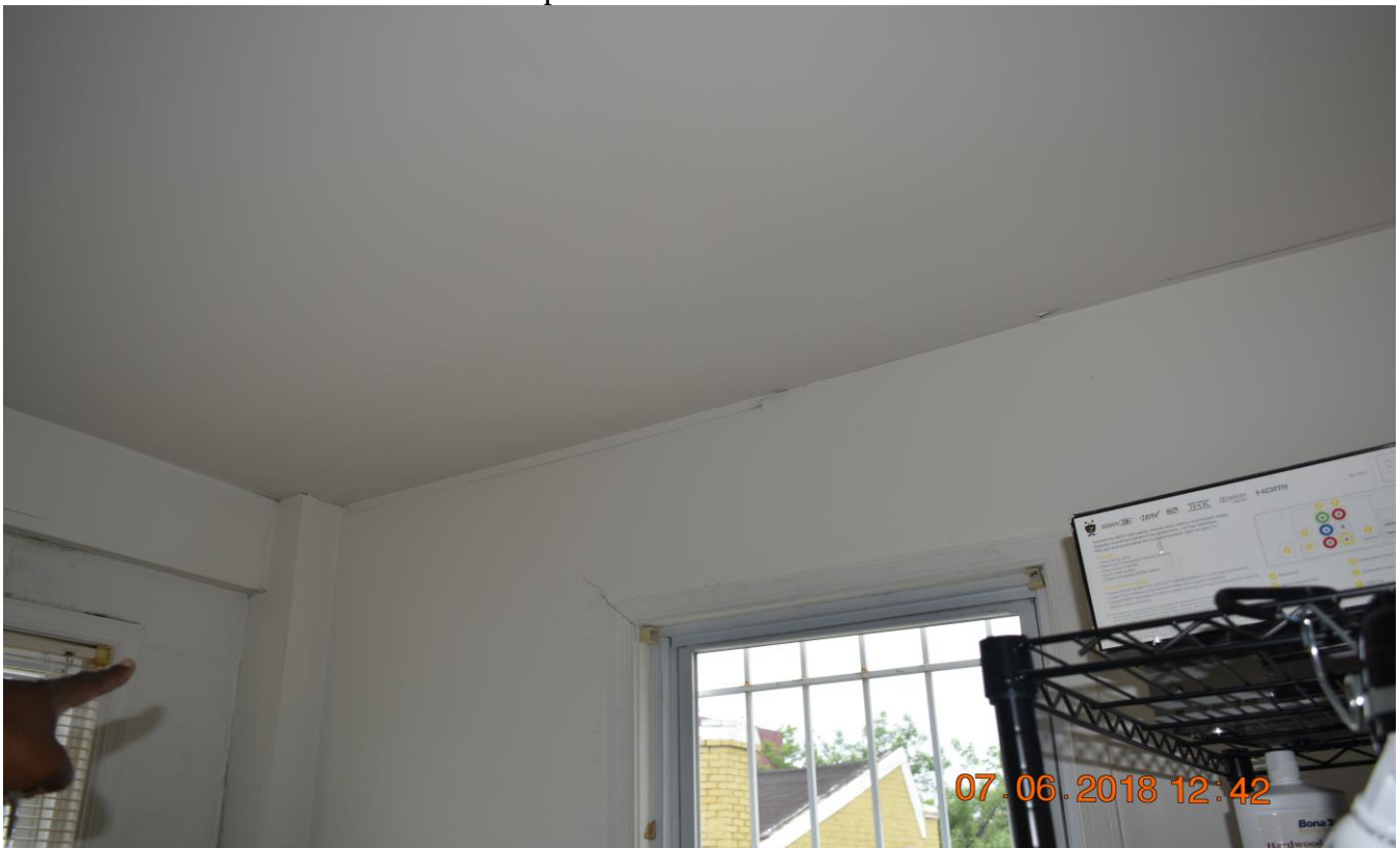
Drywall crack in window upper left corner.
