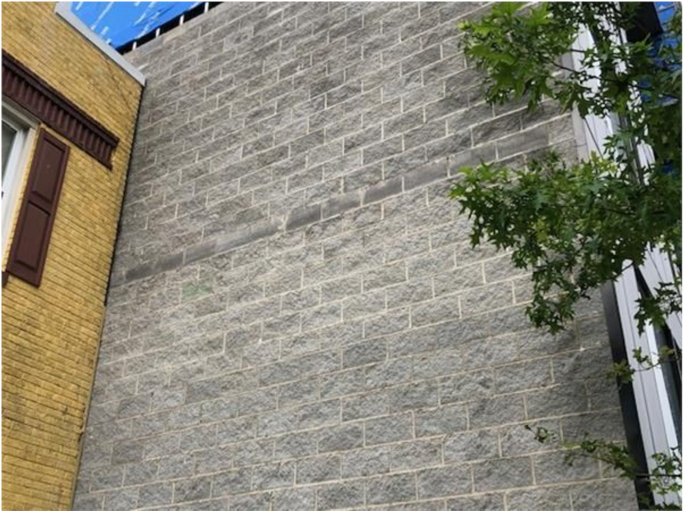
Fig 12. 770 Princeton Pl. NW@ detached adjacent wall on 3619 Georgia Ave NW.
