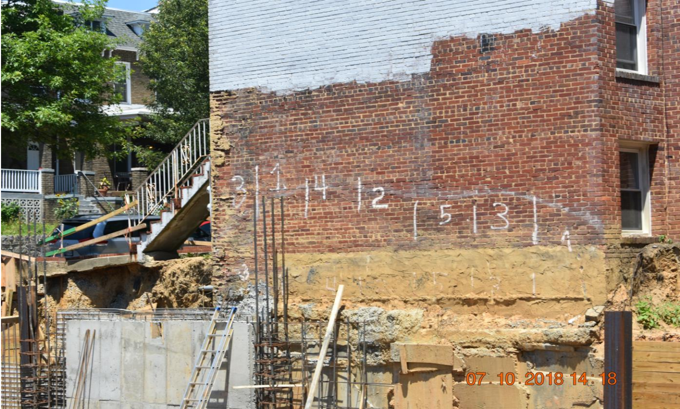
Existing landing and steps with displaced earth
