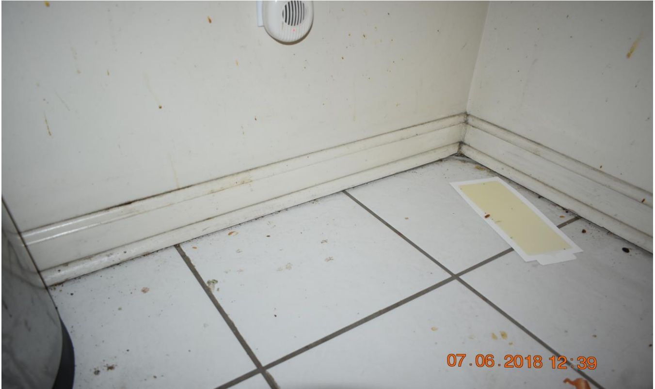
Gap at baseboard wall corner
