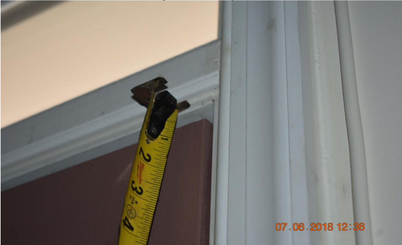
Gap at right side door jamb
