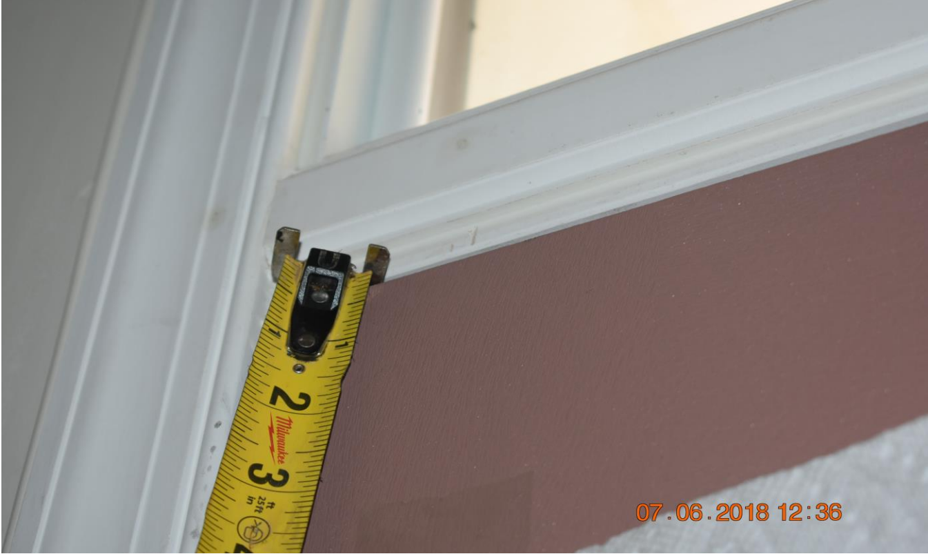
Gap at left side door jamb
