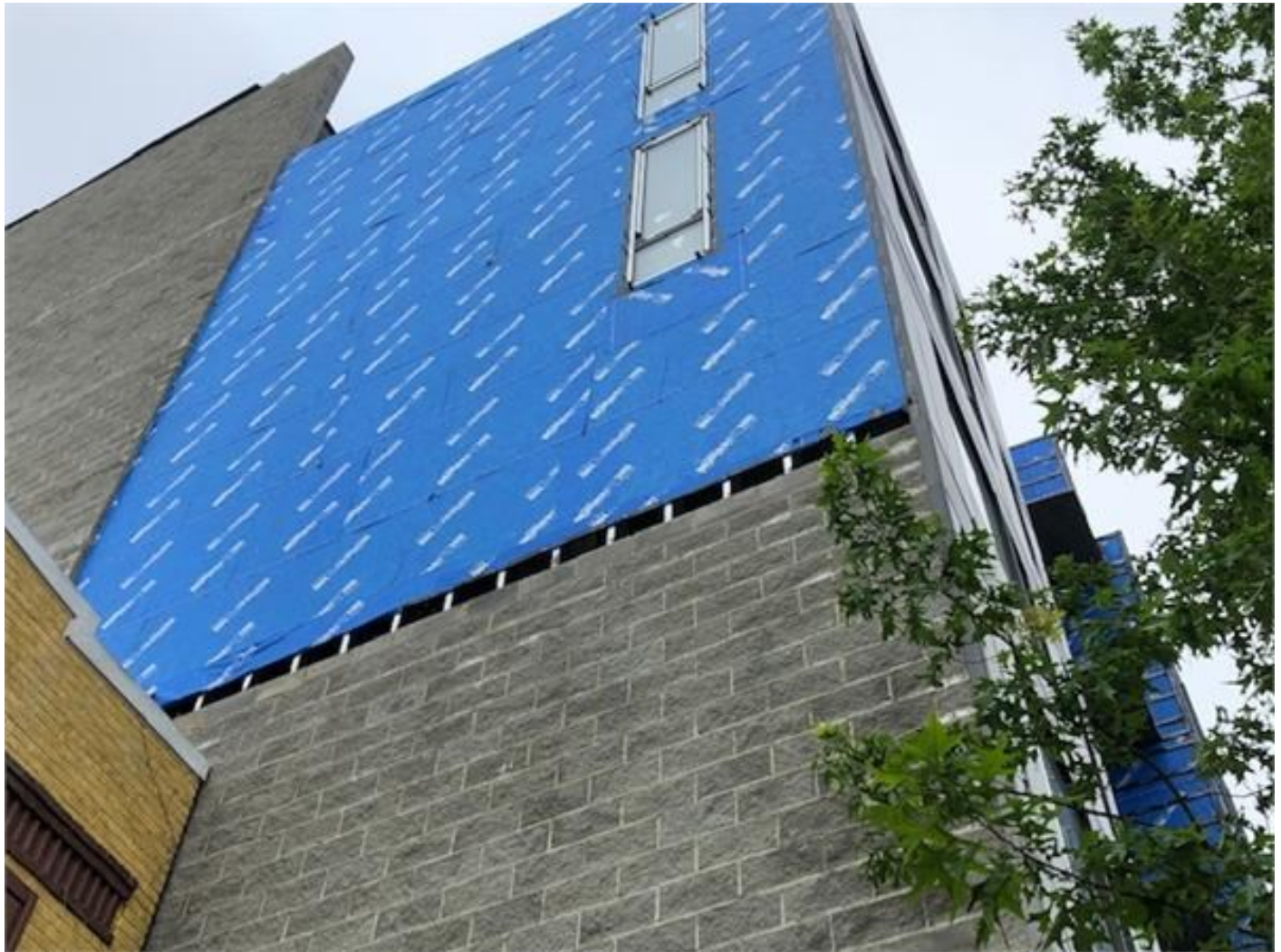
Fig 14. 770 Princeton Pl. NW@ detached adjacent wall on 3619 Georgia Ave NW.
