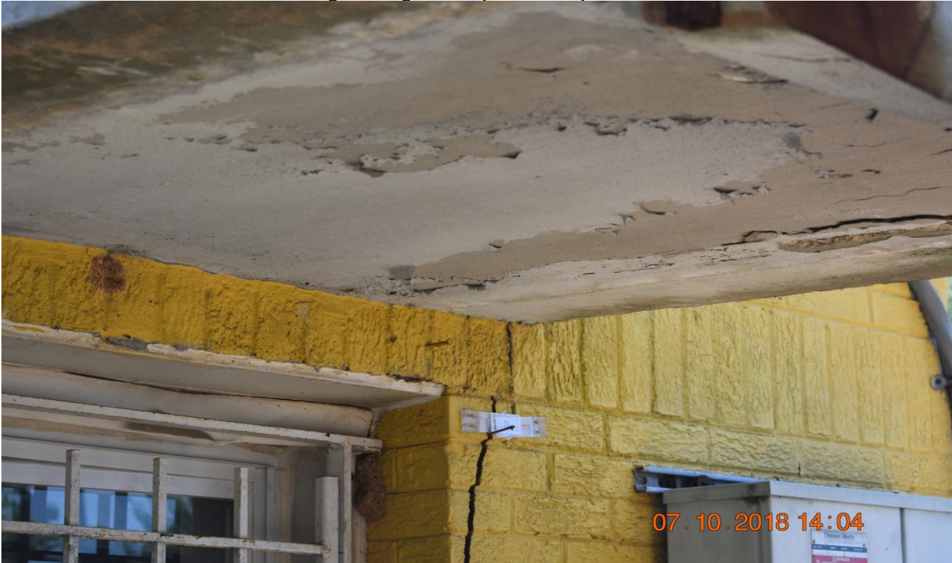
Crack on building façade wall with monitor installed
