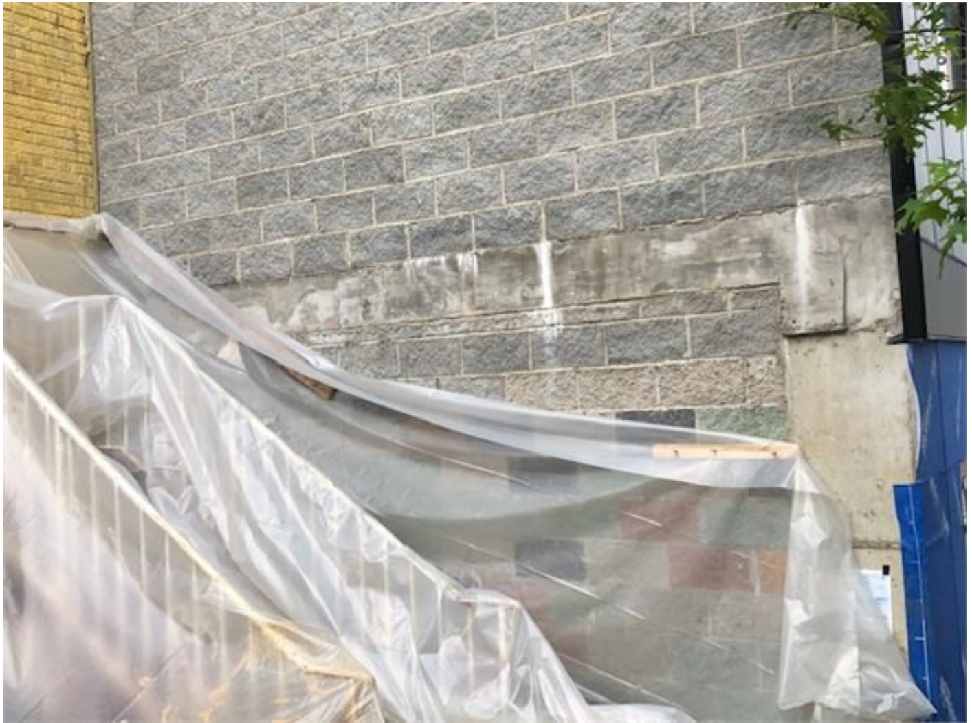
Fig 13. 770 Princeton Pl. NW@ detached adjacent wall on 3619 Georgia Ave NW.
